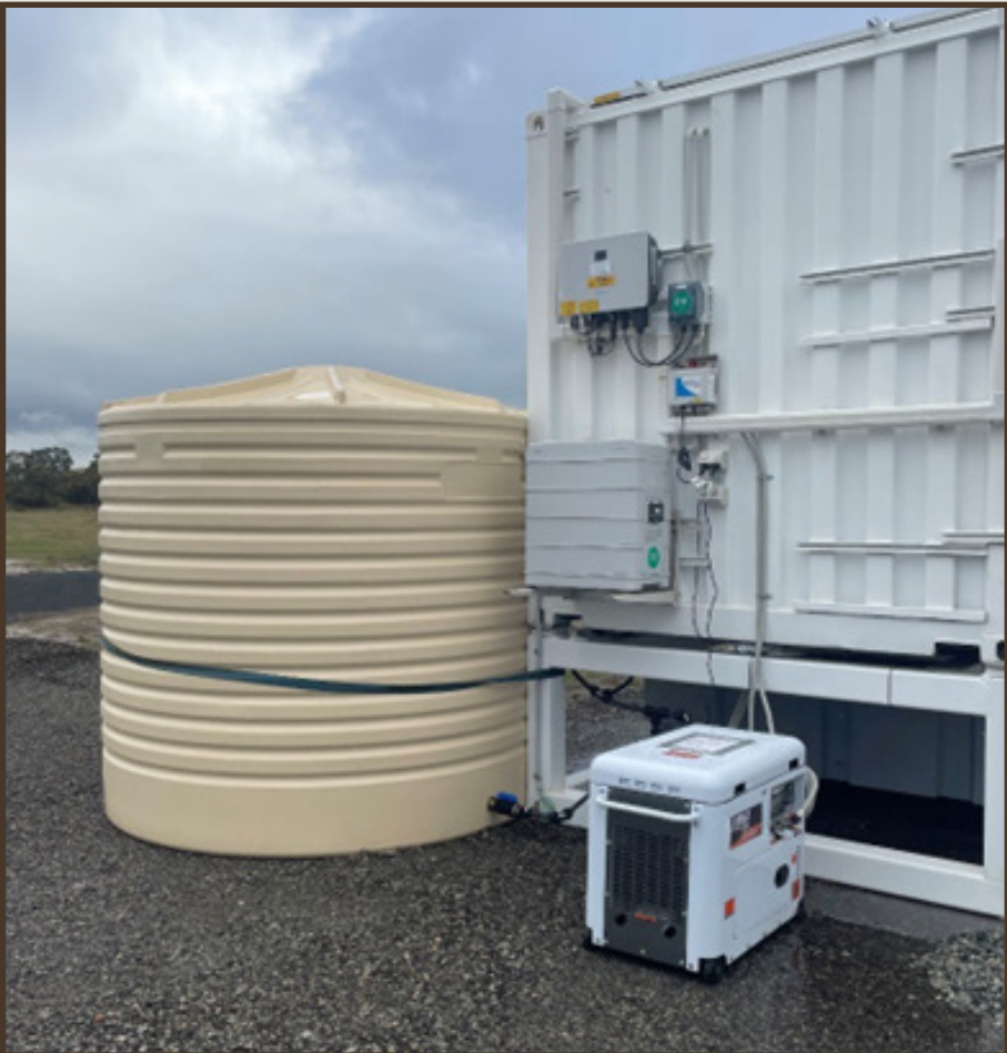
Ablution solar sea container with rainwater tank
